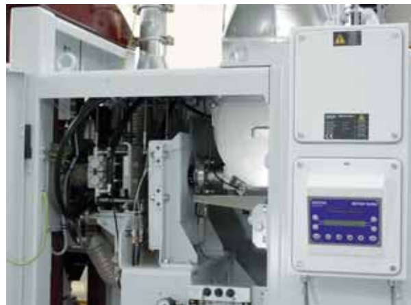
Metal detector integrated in the filling channel of the impeller packer with evaluation technology at the machine frame
